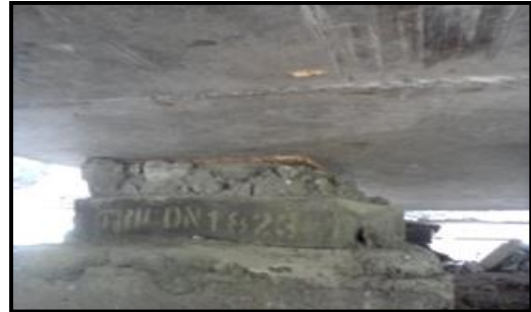
Fig. 6 – Bearing placed with top cementitious grout without proper bonding
