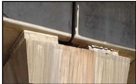
Fig. 8 – Grout so placed on pedestal it is coming out due to bond failure and train movement.
