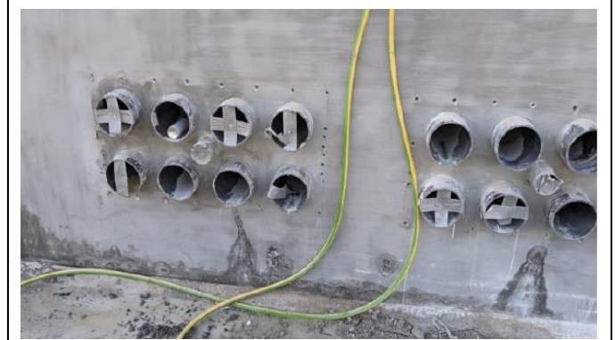
Dampness at outside basement wall
