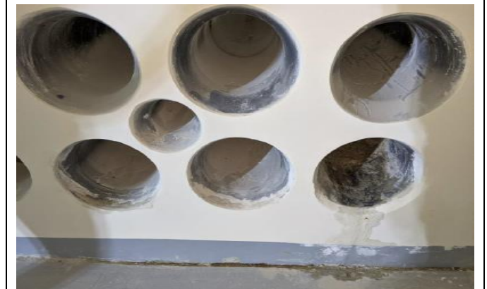
Dampness at inside basement wall
