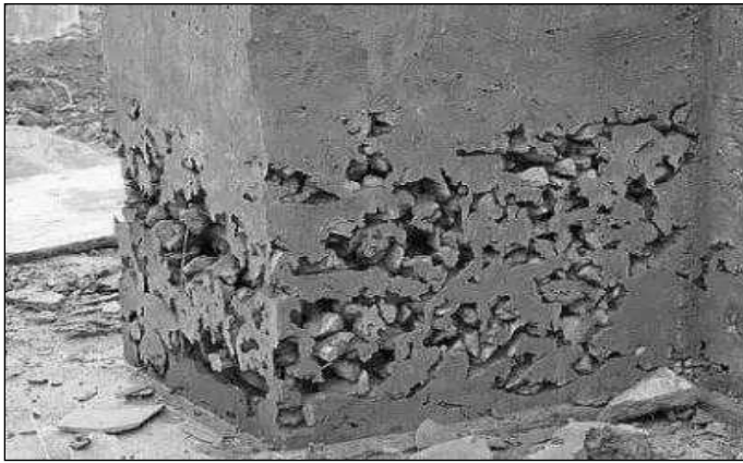
Figure 1. Anomalies during execution: voids and segregation of concrete
