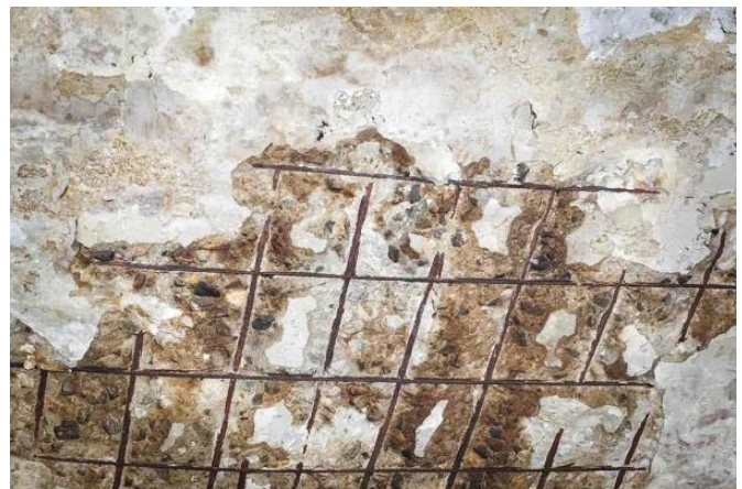
FIGURE 2. CHLORIDE DISSOLVED IN WATER SEEPS THROUGH NEGATIVE CONCRETE OR TO STEEL THROUGH CRACKS [16]
