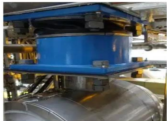
Fig 3 Installed Viscoelastic Damper
