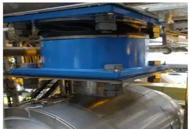
Fig 3 Installed Viscoelastic Damper
