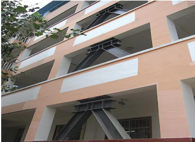
Fig 8 Metallic Yielding Damper Installed in Multistory Building
