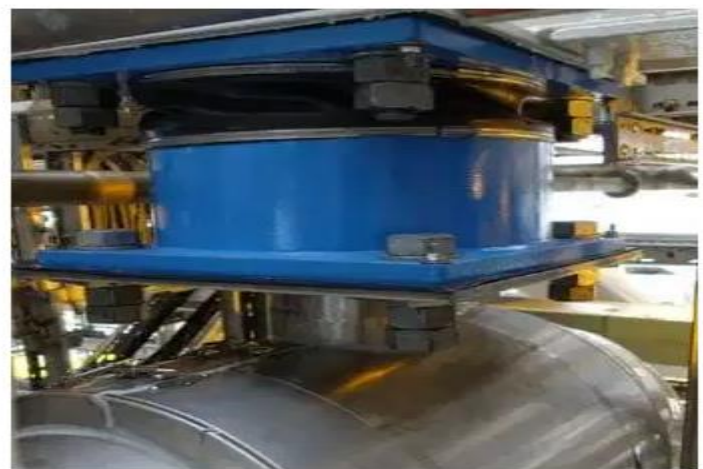
Fig 3 Installed Viscoelastic Damper
