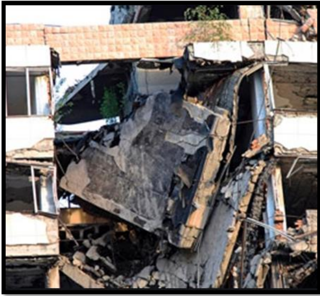
Figure 1. Damage on building due to earthquake
