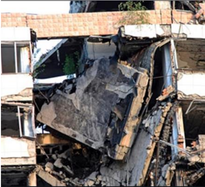
Fig 1. Damage on building due to earthquake
