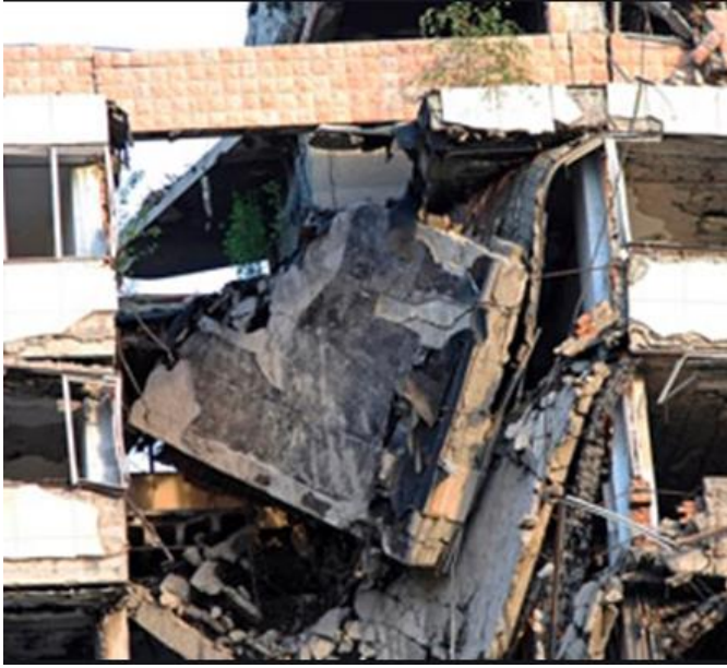
Fig 1 : Damage on building due to earthquake
